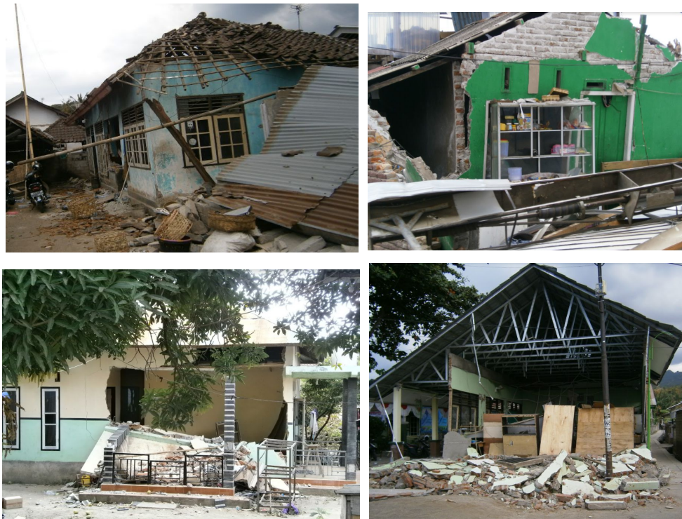
Figure. 4 Examples of poorly built houses from the Lombok Earthquake in July 29, 2018
