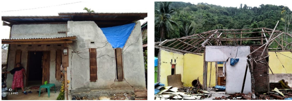
Figure. 1 Examples of poorly built houses from the West Sulawesi Earthquake in January 15, 2021
