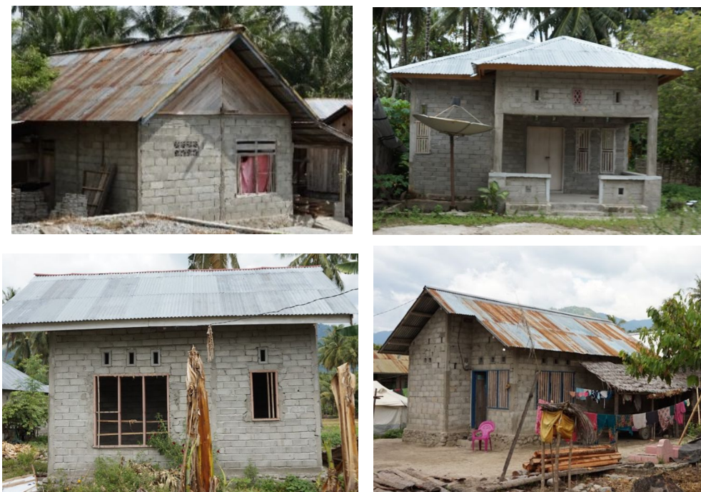
Figure. 2 Examples of poorly built houses from the Palu (Central Sulawesi) Earthquake in September 28, 2018
